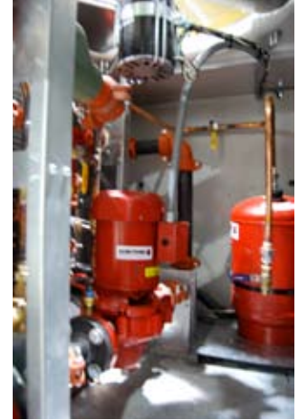
Factory Installed Pumping Package
